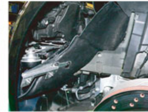
A carbon air duct is installed as well as original. Wiring of a temperature sensor is also connected as before.
